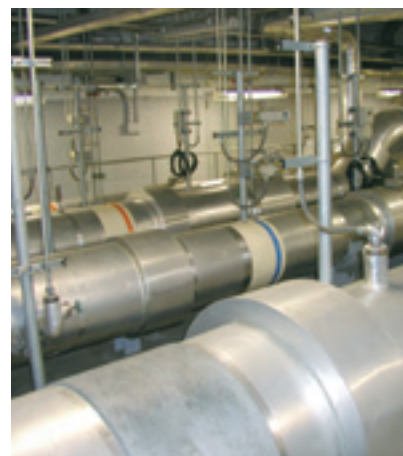
The district heating/cooling system in the Yellow Building
