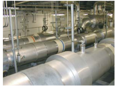
The district heating/cooling system in the Yellow Building
