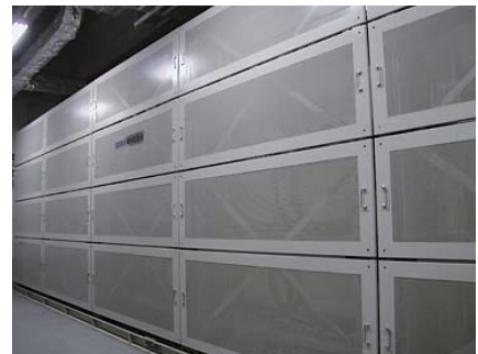
The underground NAS batteries at LaQua
