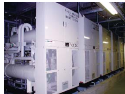
The ice thermal storage system in the Toyko Dome Hotel and LaQua
