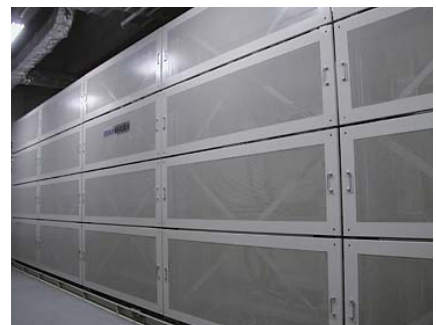
The underground NAS batteries at LaQua
