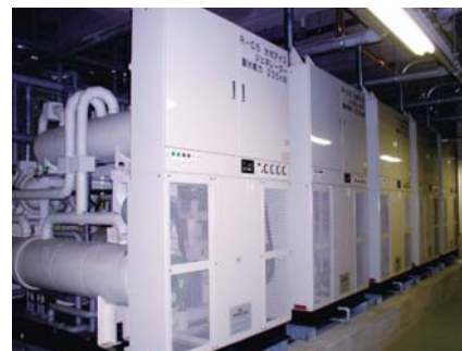
The ice thermal storage system in the Toyko Dome Hotel and LaQua
