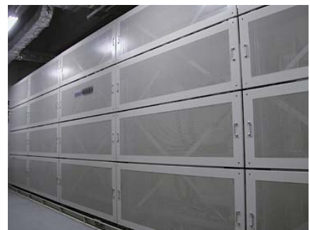
The underground NAS batteries at LaQua
